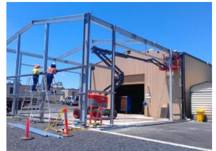
QGC-Condamine Power station
