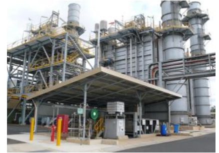
QGC-Condamine Power station Miles, QLD Design, certification, Installation
